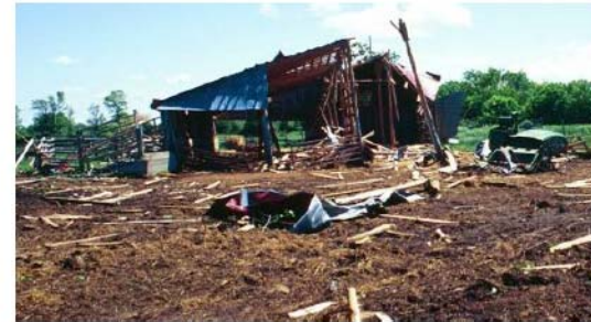
Example of SBO DOD5 with partial loss of walls and roof structure (1999 Purple Valley, ON tornado)
