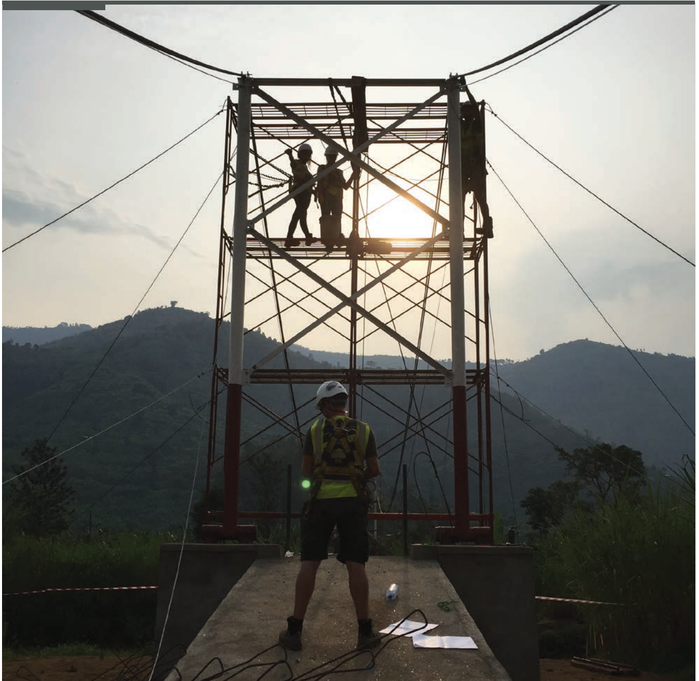
Sunset while preparing the deck hangers for installation on the Bridges to Prosperity suspension bridge in Tubungo, Rwanda © Flint & Neill
